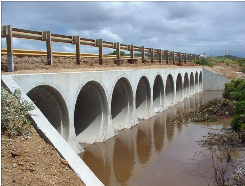
Culverts under Hamersley Drive where it crosses Culham Inlet (photo by Ralph Cooper, January 2000)
